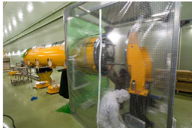
Beam pipe connection
