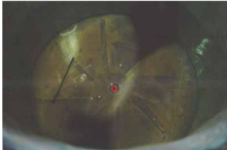
The contaminated EP acid tank
