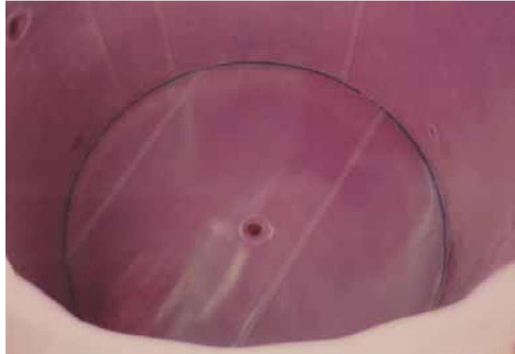
Teflon lining EP acid tank (brand-new)
