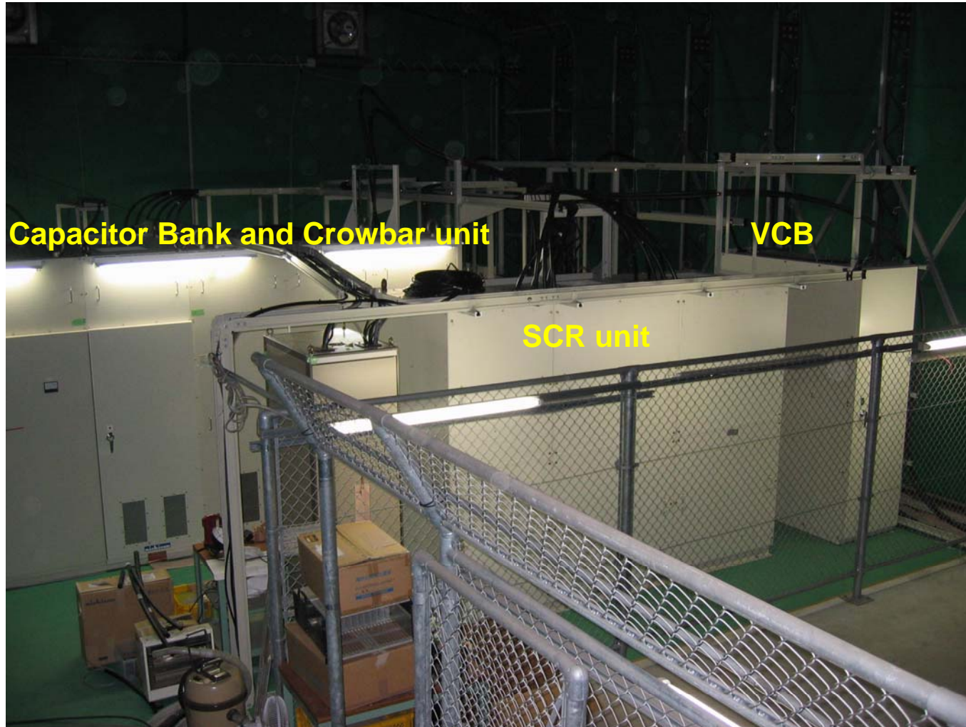
DC Power Supply(Tent House)
