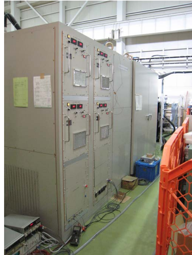
Four 50 kW switching power supplies
