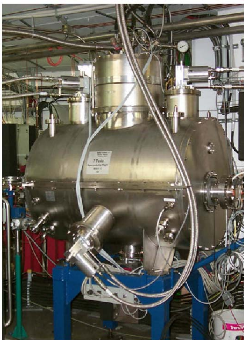
Fig. 2-4 Photo of 7 Tesla WLS inserted into BESSY-2 straight section.
