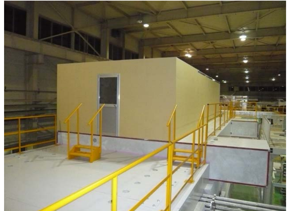
New LW hut was prepared. Waiting powers and air conditioner. Laser can be moved soon.
