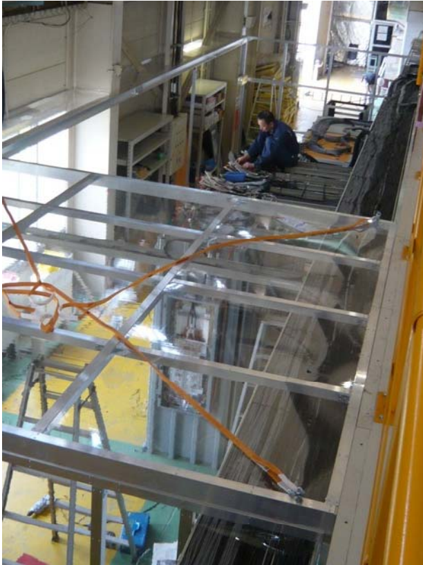
Vinyl hut for the FF beam line. HAPS, SLAC movers, BPMs, Vacuum, Timing,...
