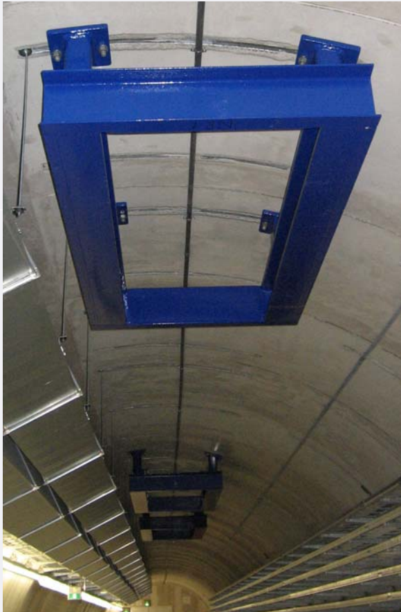
Welded ceiling interfaces - 2 per cryomodule -
