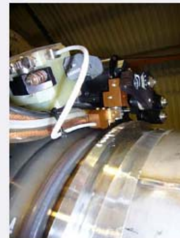
Weld tractor with special weld head for HeGRP connection, developed at Desy
