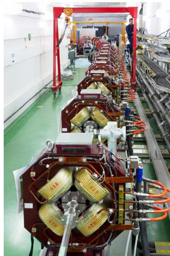
ATF2 Beam Line vacuum pipe connected in October
