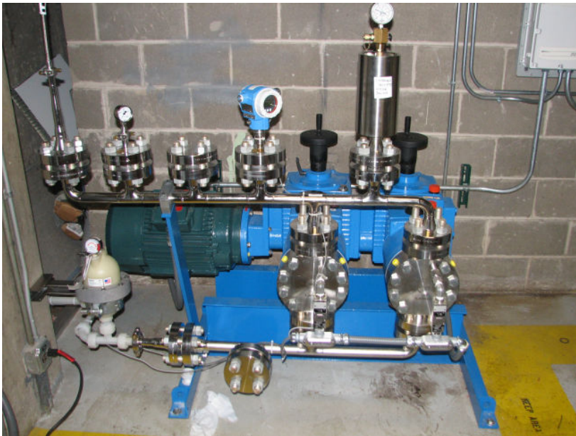
LEWA HPR pump and manifolds.
