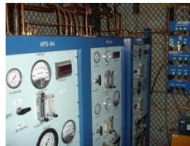
Gas delivery to 6 locations
