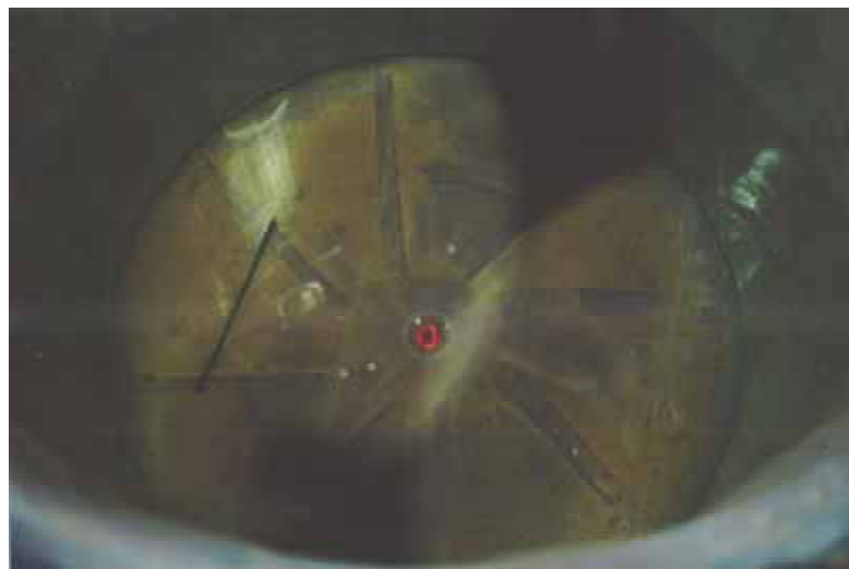
The contaminated EP acid tank
