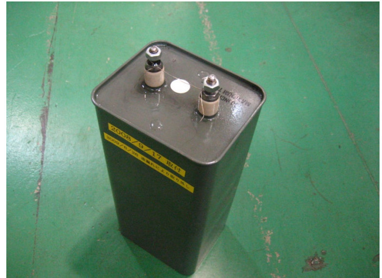
oil leaking capacitor
