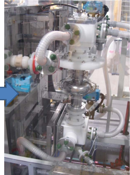
Drain EP acid for 10 min. Then UPW rinse starts.
