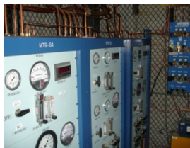
Gas delivery to 6 locations
