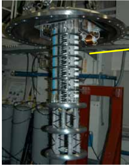
550kV Cockcroft Walton power supply
