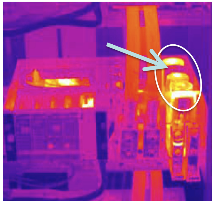
One of the four filter capacitors failed open circuit and is running cooler than the others. This causes stress on the other caps, which will eventually fail and cause downtime.
