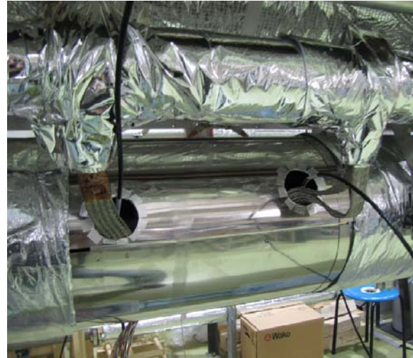
Magnetic shield between the AES004 and ACC011
