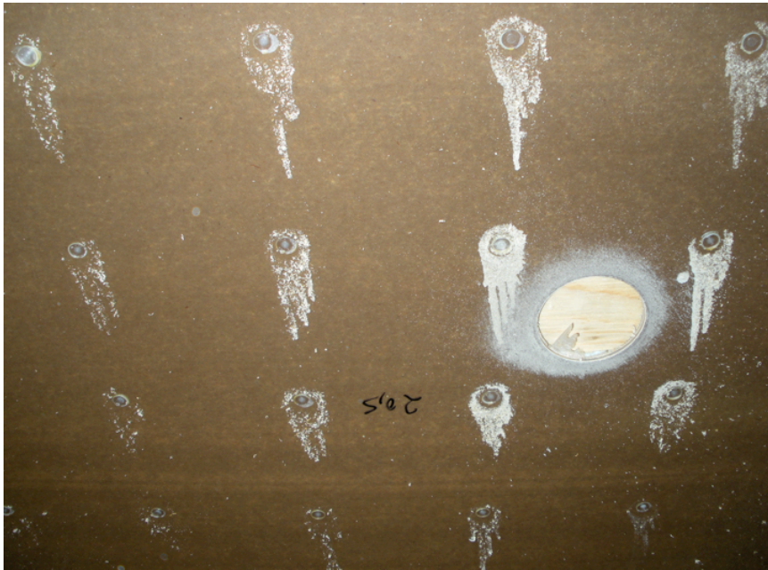
Drain Marks Around Buttons
