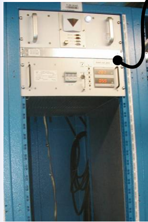
280V bulk supply in USA15
