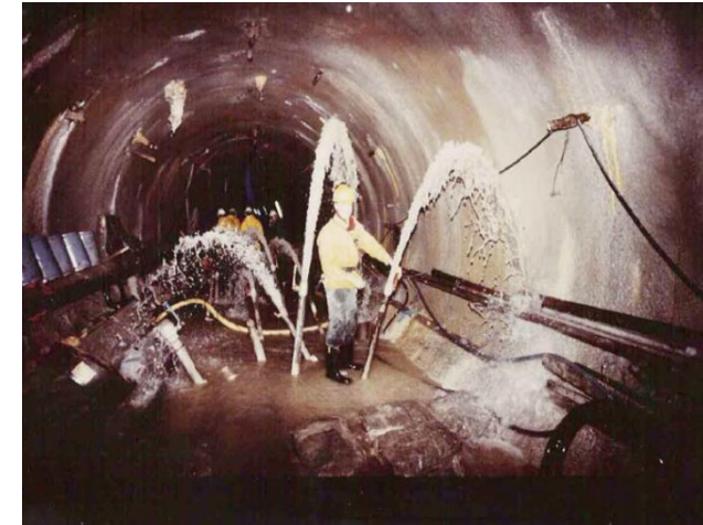
LEP tunnel collapse
