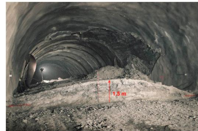
Example of tunnel invert heave Chienberg tunnel, Switzerland
