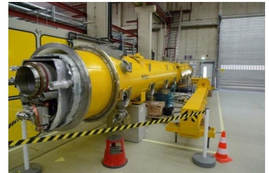
12 m Cryomodule for Euro-XFEL PXCEL1 in FLASH; 58 ordered for XFEL
