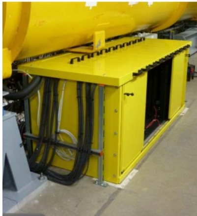
Injector-like LLRF racks in FLASH tunnel
