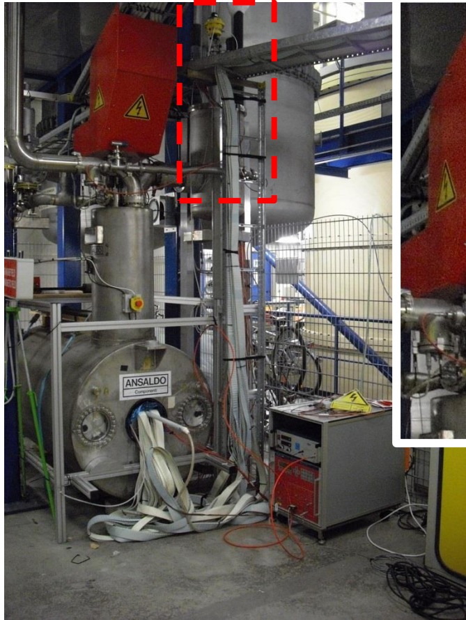
Magnet Outlook at Cryogenic Hall
