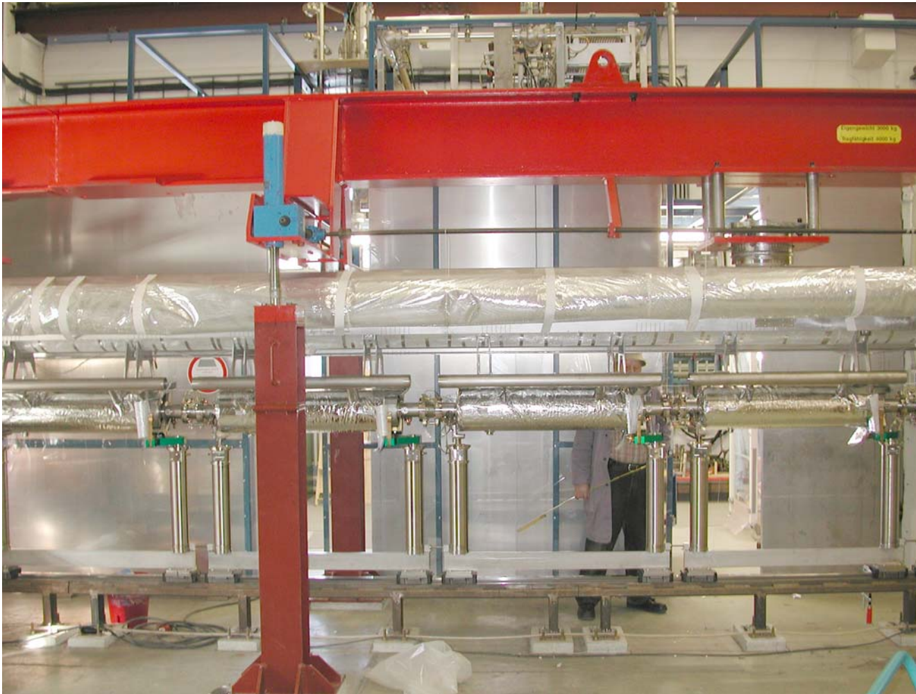
String in the assembly area
