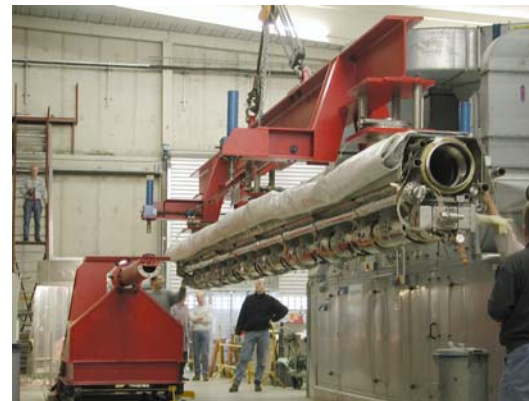
Assembly outside cleanroom
