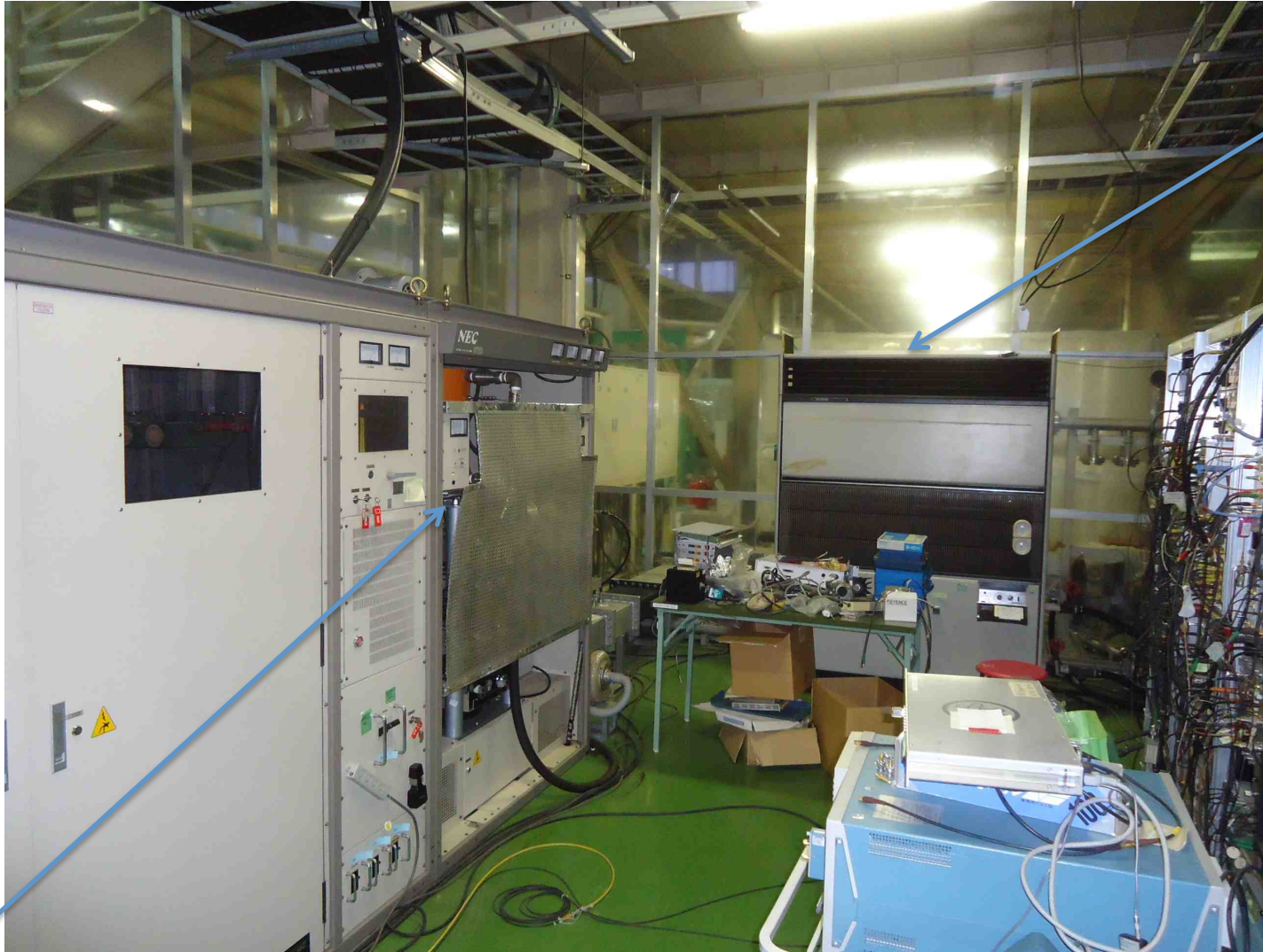
Air Conditioner for Klystron
