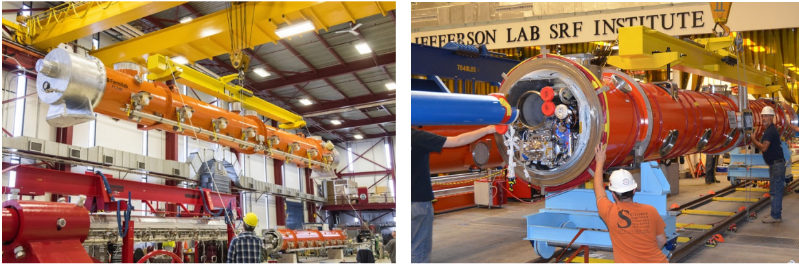
Figure 4.28: View of some of the cryomodule assembly facilities at Fermilab (left) and Jefferson Lab (right).
