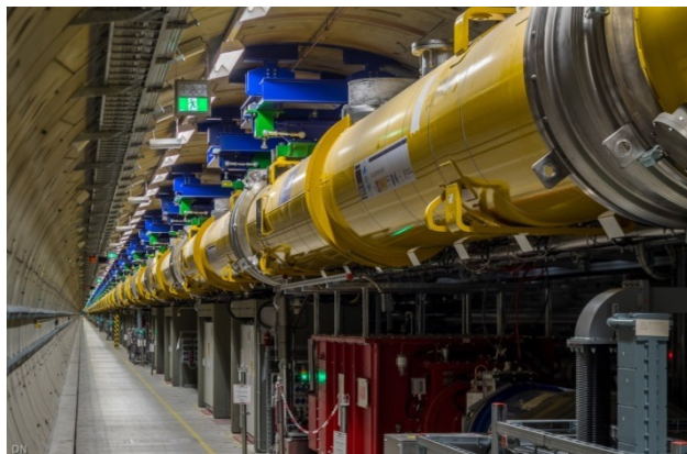
Figure 4.7: View of installed cryomodules in the tunnel of the E-XFEL [37].
