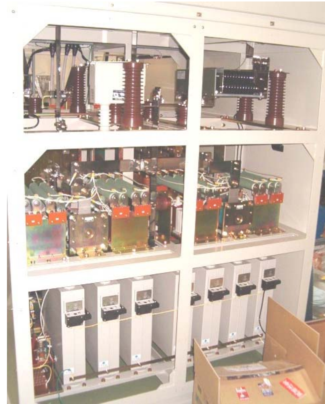
Pulser Unit for a Pulse Transformer Modulator
