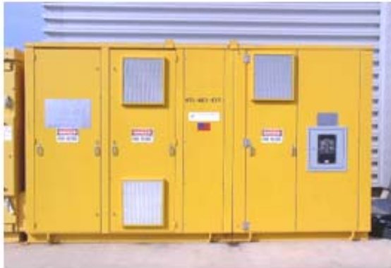
RECTIFIER TRANSFORMER AND FILTERS
