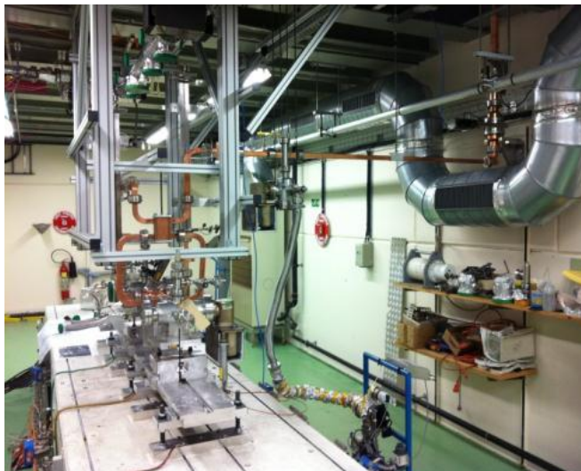
XBox1 at CERN operational with SLAC klystron
