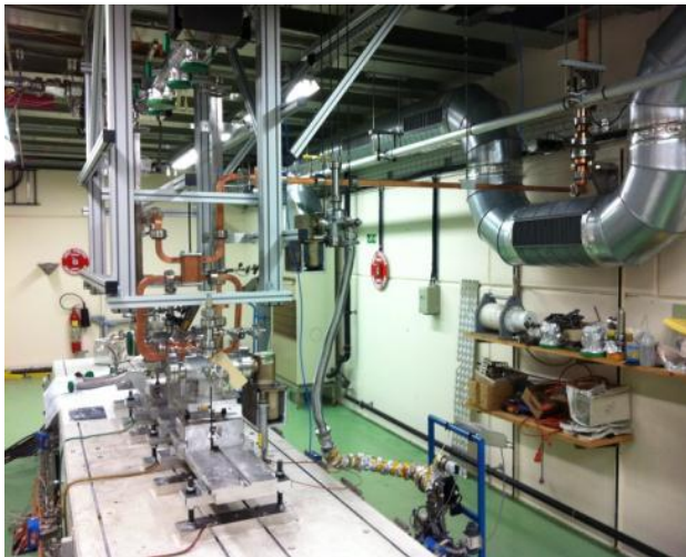
XBOX1 at CERN operational with SLAC klystron
